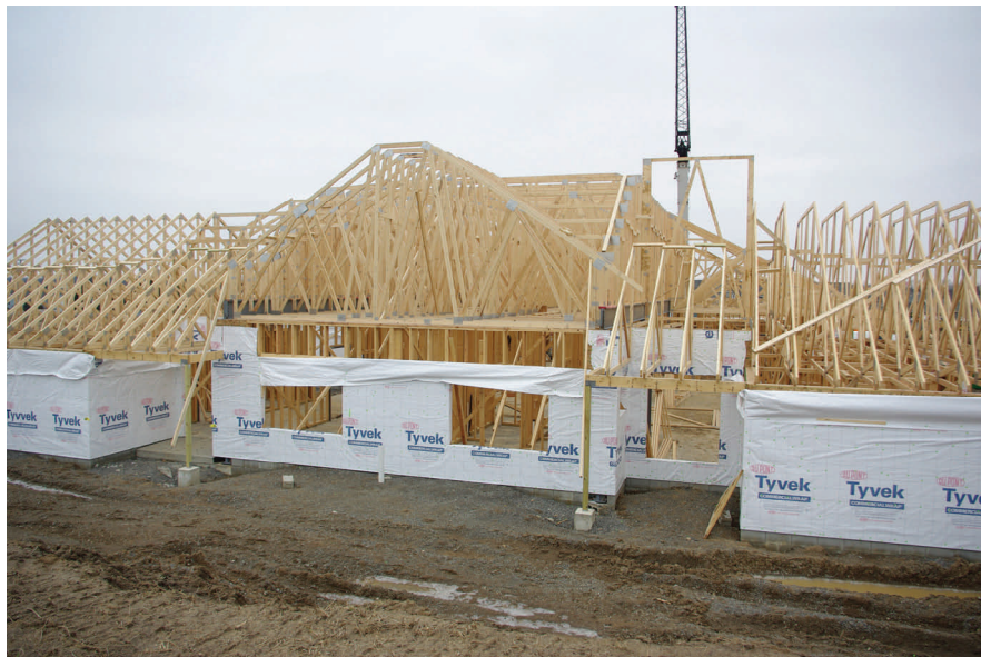
Signs of Progress: The trusses are up on House "B." Trusses on House "A" will go up soon. (Photos by Kris Reese)
